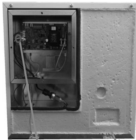
BT15 connector Insulation BT15 is in the back.
