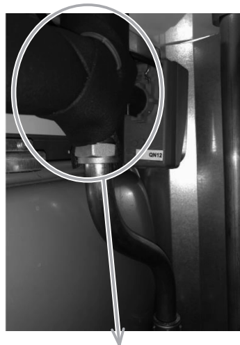
Insulation and valve from QN12
