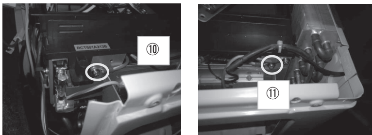
Fig.5 Earth cable of control box
